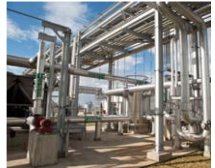
Sanofi is committed to optimizing our energy consumption and energy security for all our business activities – utilities network area of Sanofi Pasteur, Toluca, Mexico.
